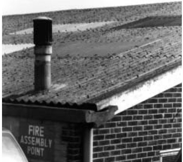
11c Asbestos cement external flue, rain water gutter and profile roofing sheet.
