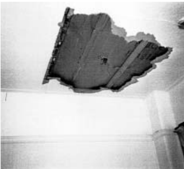
1a Acoustic insulation in a ceiling void with a 'Jiffy bag'-type construction, with paper container punctured for electrical wiring.
