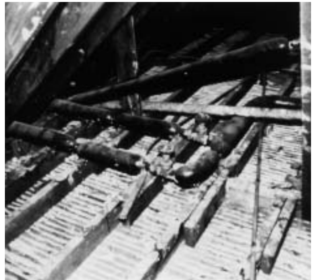
3a Asbestos-insulated water pipes in a loft, sealed and in good condition.
