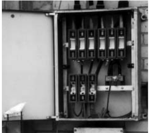
18c Asbestos tape flash guards in a fuse box.
