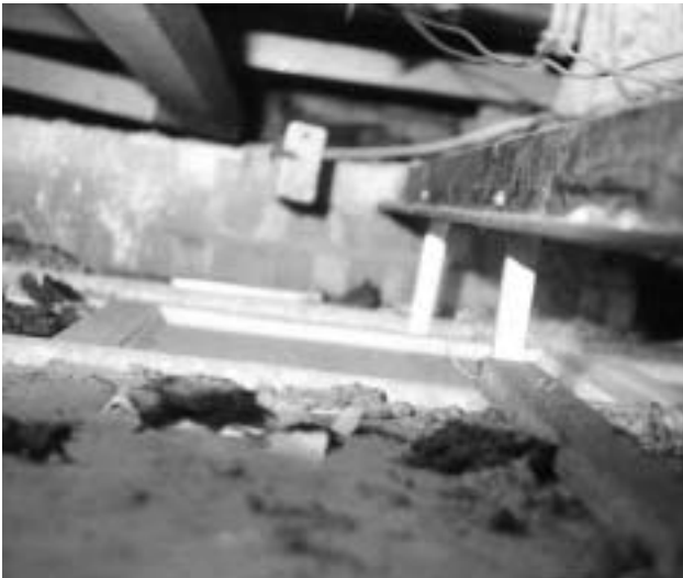
20d Sprayed asbestos debris released onto a suspended ceiling from cable installation work.
