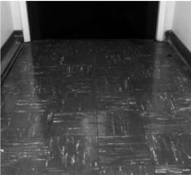
14a Asbestos-containing vinyl floor tiles.
