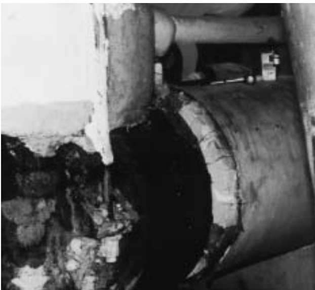
3g High-pressure steam pipes in a power station with a 'Bulldog' finish over 'Caposil' insulation blocks.
