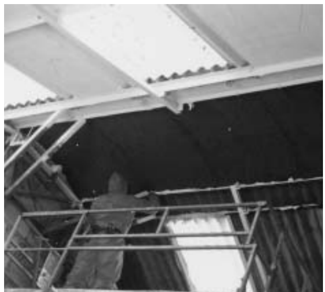
2d Sprayed crocidolite asbestos (100 mm thick) applied as thermal insulation to the underside of an asbestos cement roof. From top to bottom, the encapsulated spray, the spray without encapsulant and removed spray from the A/C cement sheets.
