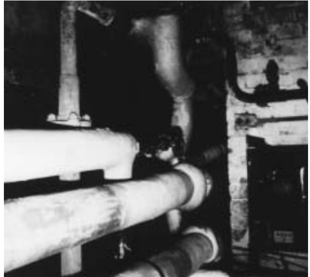
3d Asbestos pipe lagging on central heating pipes at the entrance of an underground crawl tunnel to adjacent premises.
