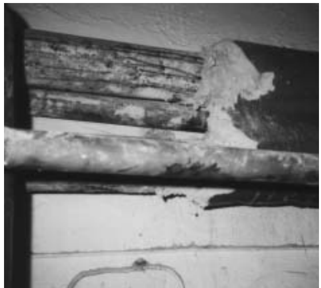
3i Example of hand-applied 'hard set' insulation, partially removed from a pipe.
