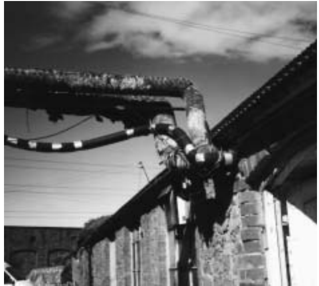
3h Badly degraded external asbestos-lagged pipe in an industrial plant, with asbestos rope wound around the bends.
