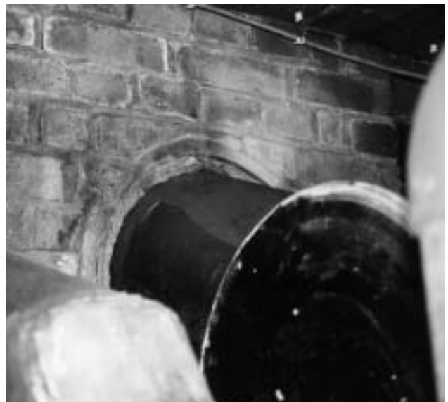
8e Asbestos rope used as packing/seal where pipe passes through a wall.
