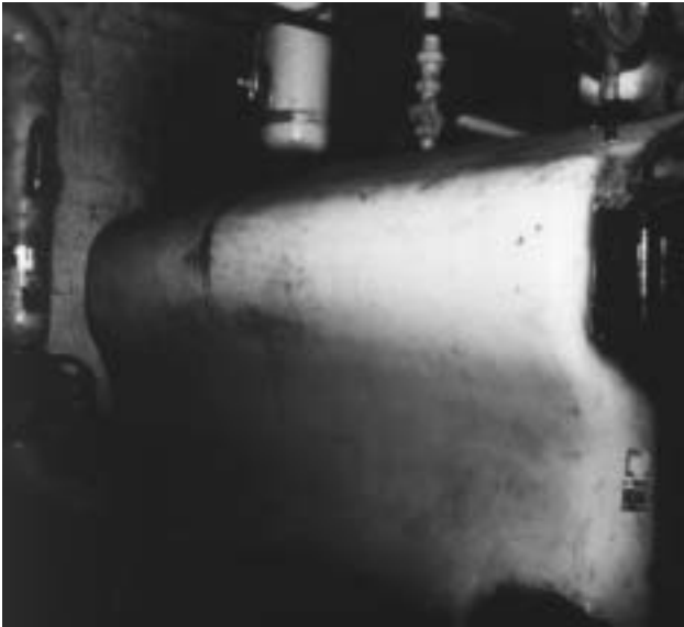
3f Asbestos-lagged boiler with a hard plaster coating.
